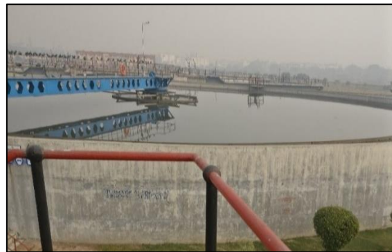
Fig 6: Aeration Tank of Okhla Plant using ASP
